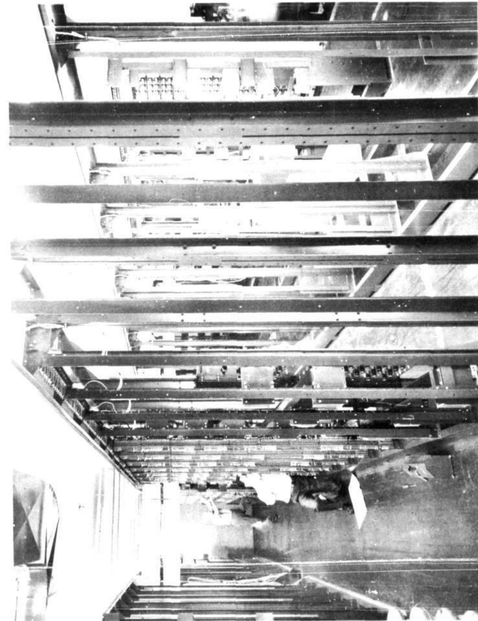
FIG. 2. POWER DISTRIBUTION HARNESES, TERMINAL STRIPS, AND FILAMENT TRANSFORMERS ARE BEING INSTALLED IN THE COMPLETED RACKS
