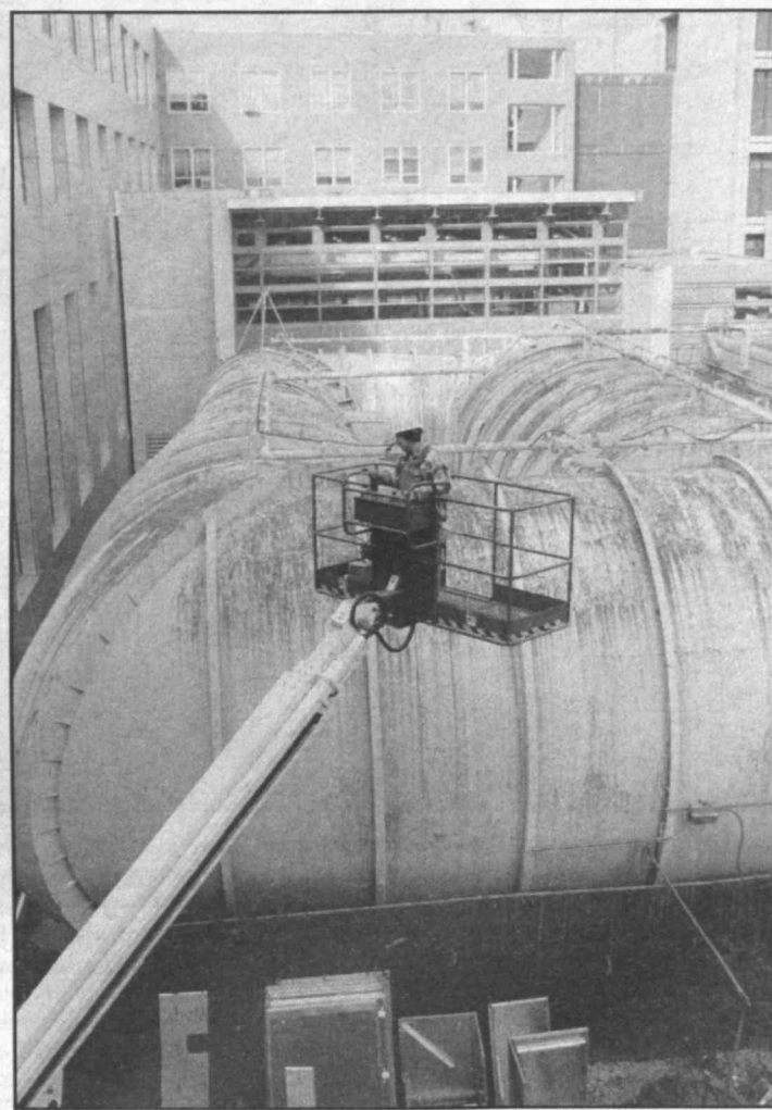
This workman is getting a bird's-eye view of the Wright Brothers Wind Tunnel, with Building 33 in the background. Photo by Donna Coveney
