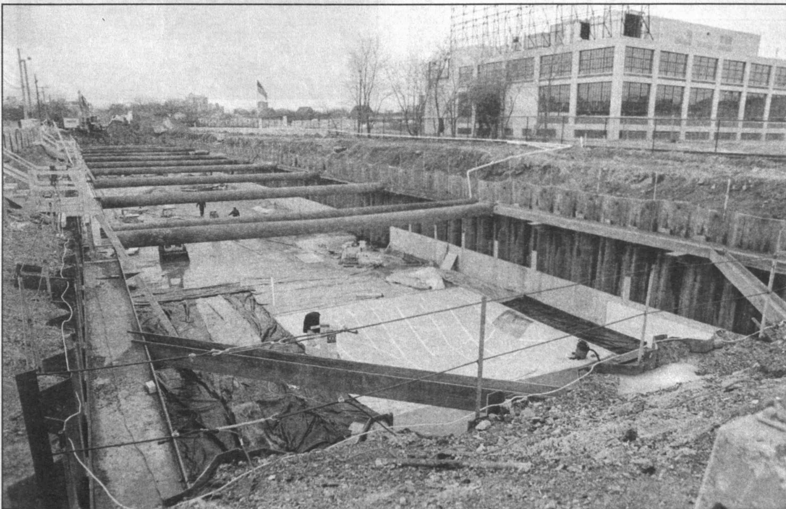
Despite frigid temperatures and rock-hard ground, the basement of Simmons Hall has taken shape on Vassar Street. Photo by Donna Coveney
