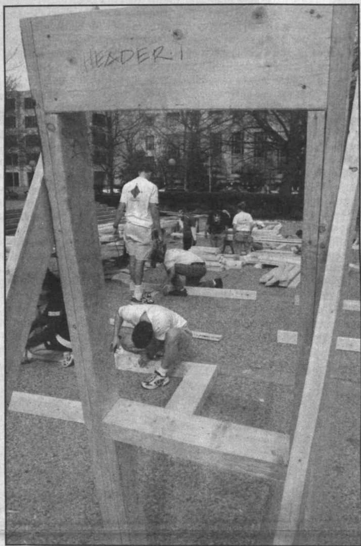
Students and staff volunteering for Habitat for Humanity built frames next to the Student Center for houses that will eventually appear in Roxbury and elsewhere. See page 8. Photo by Gábor Csányi
