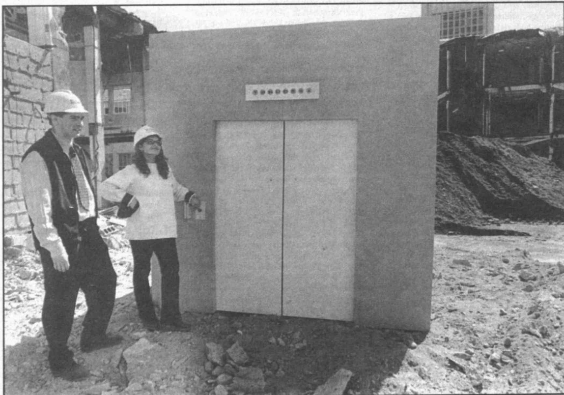
Demolition workers Steve Mahoney and Frances Bonet gamely push the button on an "elevator" they discovered amid the rubble that was Building 20. Photo by Donna Coveney
