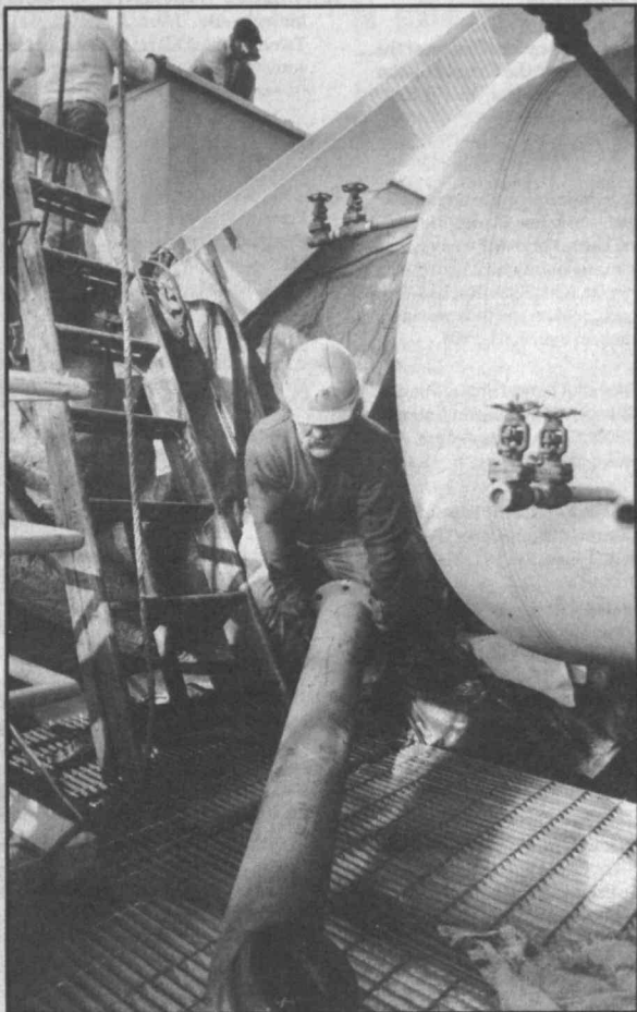
John Hogan of Pipefitters 537 moves a pipe on the top floor of the building as coworkers weld behind him.
