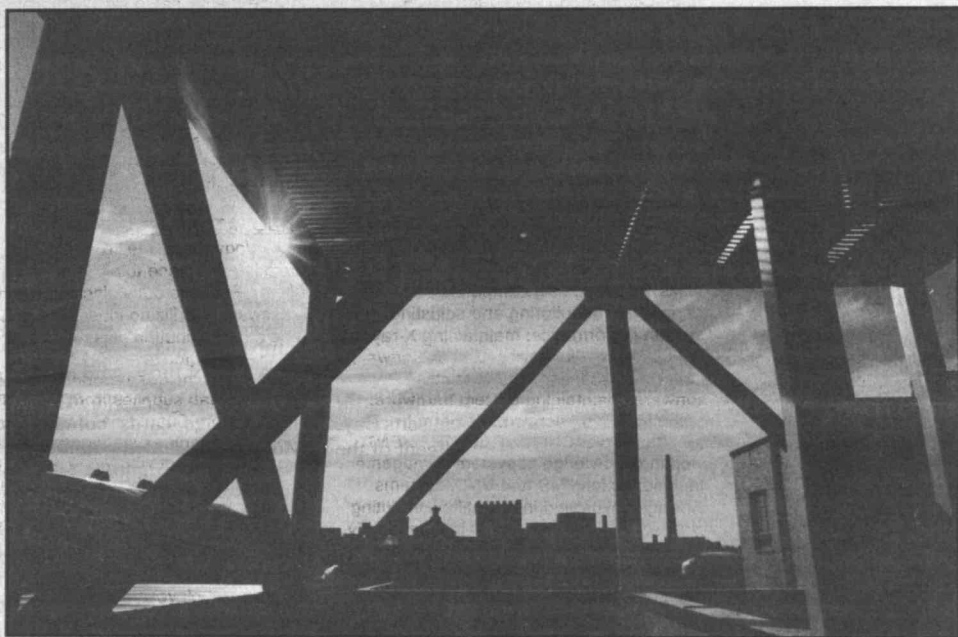
Exposed beams on the unfinished top floor of the new plant frame the Cambridge skyline and the afternoon sun.
