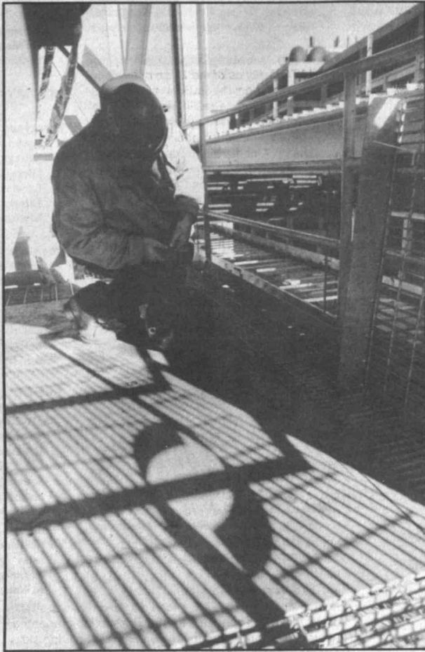
A pipefitter works high above the campus amidst shadows resembling a musical staff.
