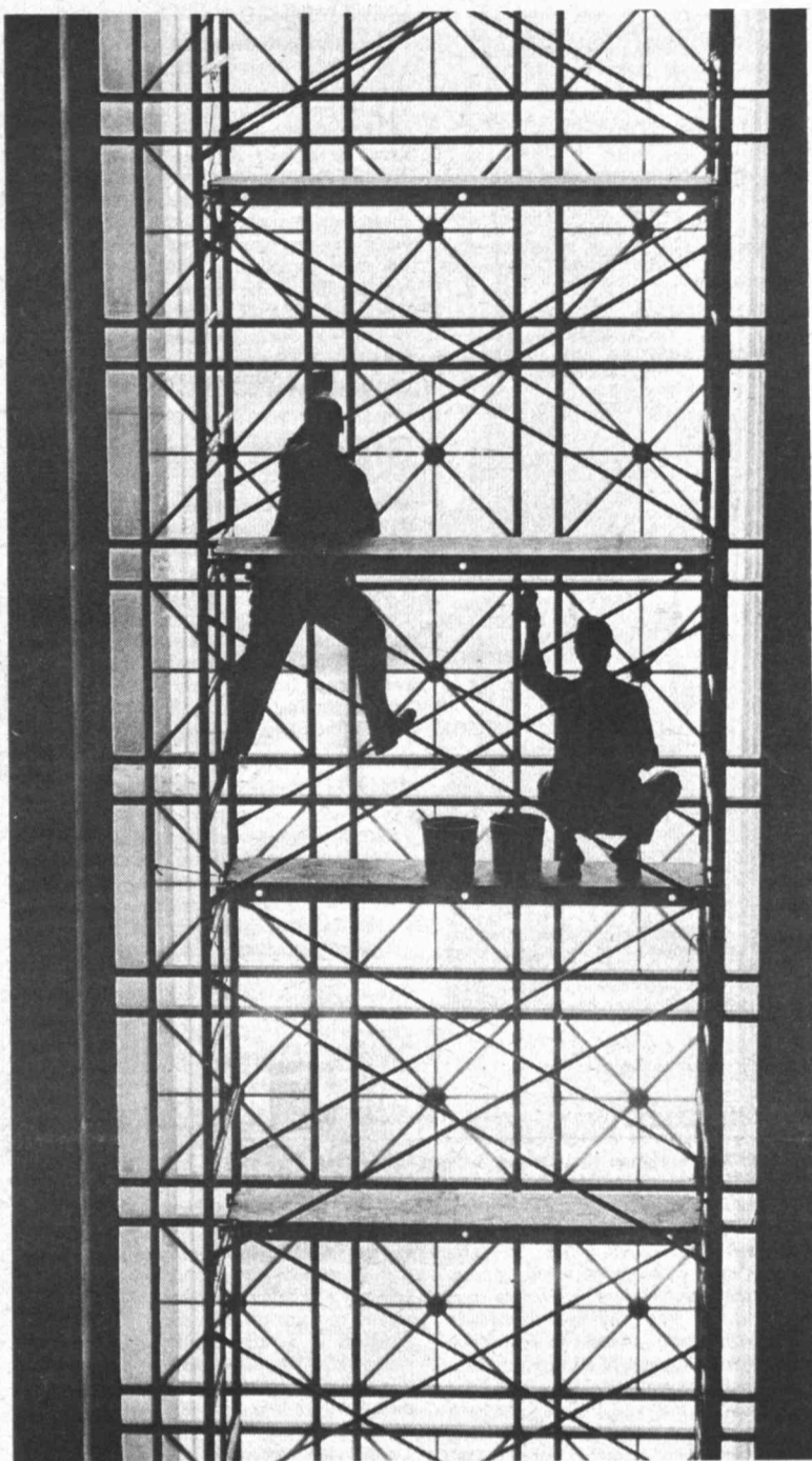
CLEAR VIEW SPECIALISTS —The four-story high windows flanking the pillared entrance to MIT's William Barton Rogers Building at 77 Massachusetts Ave., are cleaned of a long winter's grime by William Canty, left, and Mel Burnham, both of Charlestown, employees of Arro Contracting Co., Inc., of Charlestown, MIT's window cleaner since 1947. The building, MIT's main entrance, is named for the founder of the Institute. Phil Mack, who heads Arro, said there are more than 100,000 lights (windows) of glass in Buildings 1 through 11 alone.
