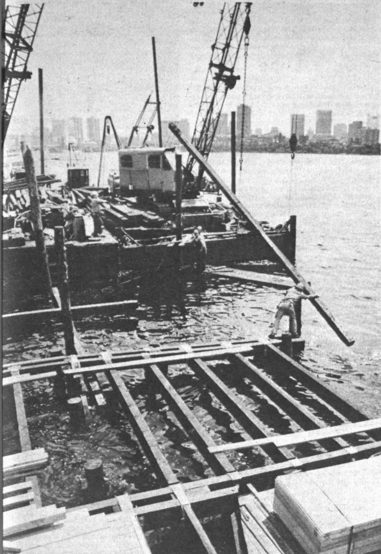
SAILING FACILITY GROWS —Heavy support timber is lowered into place at MIT's Sailing Pavilion which is being expanded. The construction work will increase the pavilion's capacity by about 25 percent and add 120 feet of dock space. Mooring slips and boat lifts also are being constructed. The lifts will allow boats to be hauled out of the water for storage or for towing to off-campus races. The MIT sailing program, oldest collegiate program in the nation, dates to 1936. George Warren Smith of Rockport, Mass., Class of 1926, heads the Sponsoring Committee for rejuvenation of the Sailing Pavilion. Nearly $285,000 in gifts and pledges has been raised to date.
