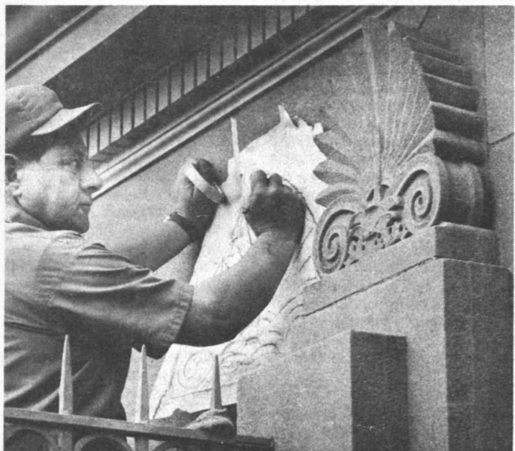
STONE CUTTER Edward J. DiRocco traces design of limestone ornament atop pier at Sailing Pavilion. Tracing will be used when new limestone ornaments are cut for Sailing Pavilion expansion.
