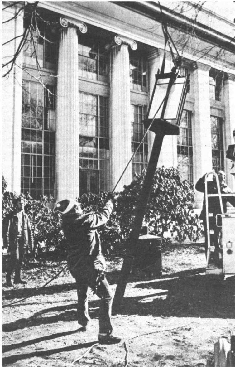
Workmen carefully lower one of the lights in Killian Court. The fixtures are to be restored and mounted on new poles. See story, page 8.
