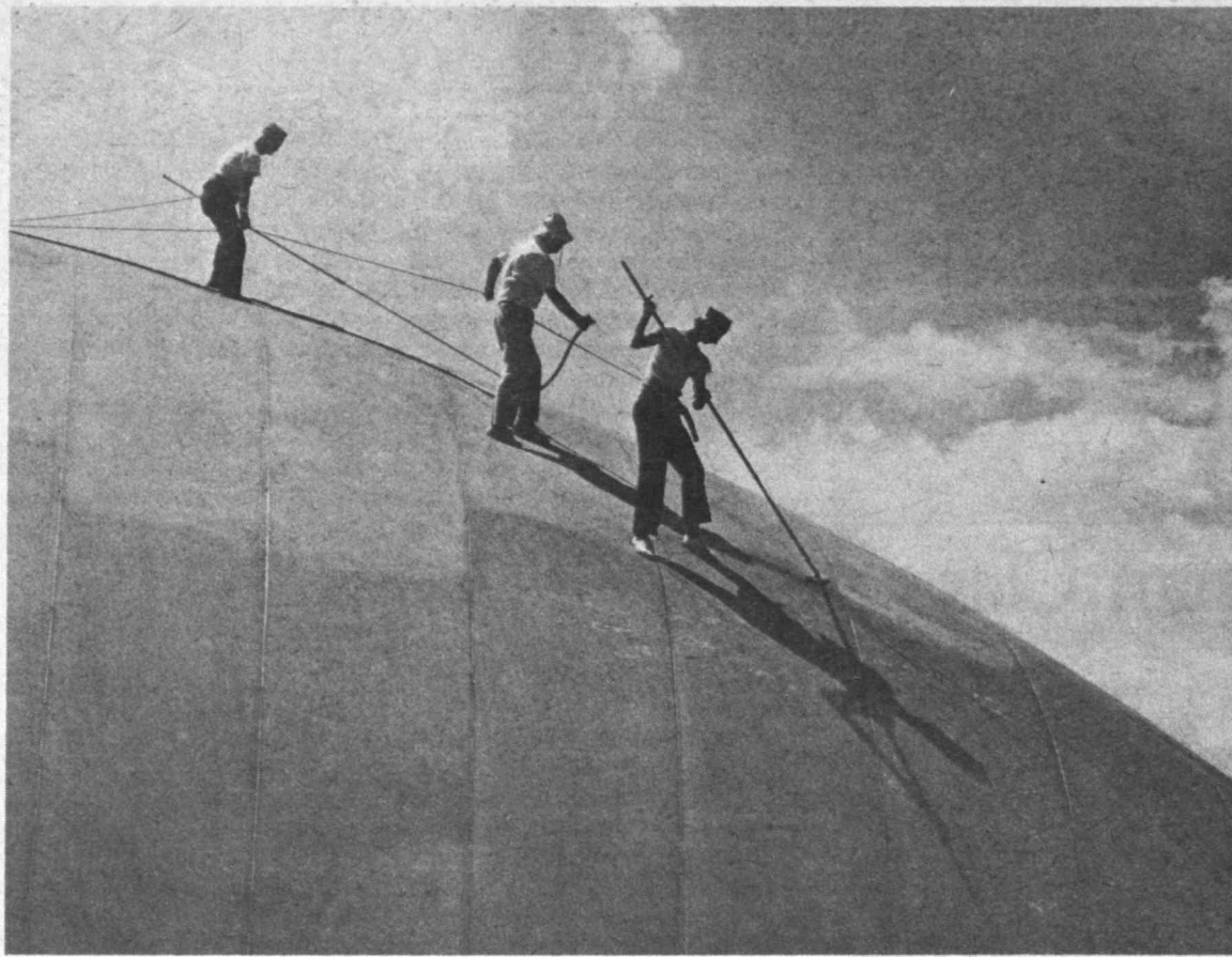
CLOUD CLEANING. Workmen at MIT appear to be lost in the clouds while they wash the outer surface of MIT's J.B. Carr Indoor Tennis Center preparatory to painting. The air-inflated structure formed from heavy-duty fabric is 212 feet long, 120 feet wide and 40 feet high and covers four tennis courts. Dedicated in 1971, it was the gift of Mr. and Mrs. J.B. Carr of
