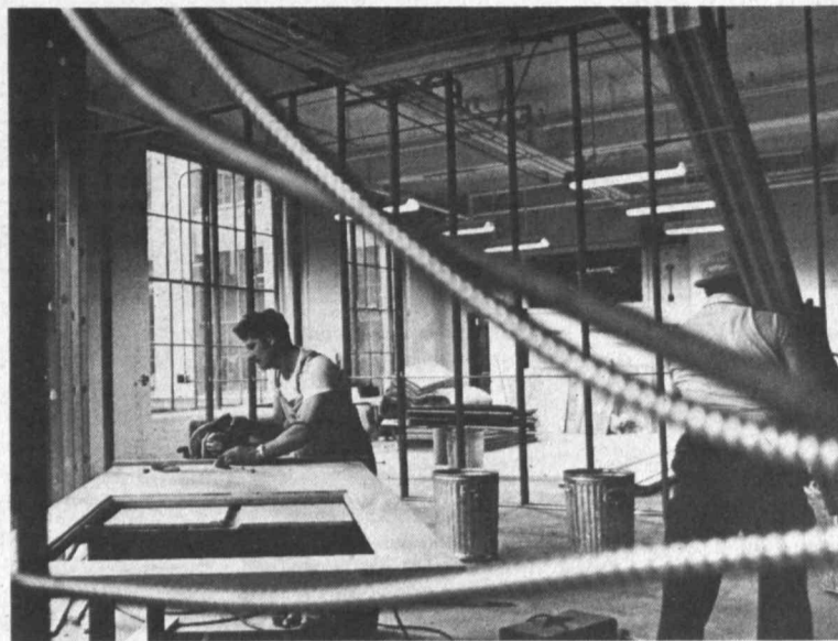
Believe it or not, this space in building 4 will shortly be ready for business as a new classroom. --Photo by Margo Foote
