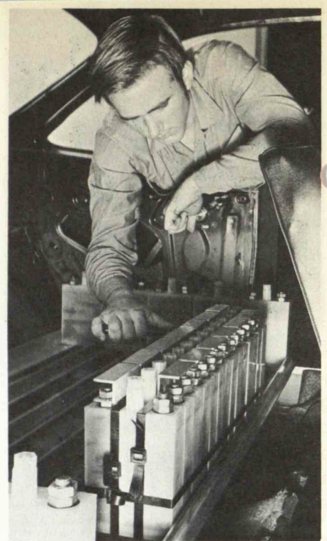
The first of ten ranks of batteries is installed in the back seat area.
