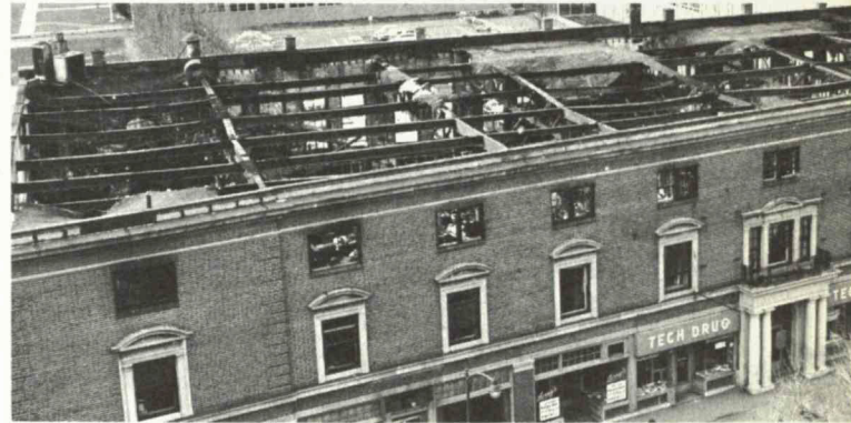
Tech Block after fire
