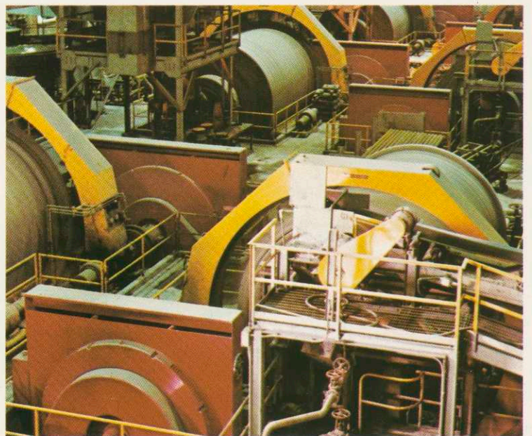
Grinding mills of various types are selected to suit projects. Rod and ball mills of this iron beneficiation plant, Ontario, Canada, are an example.
