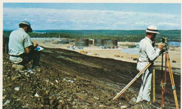
Engineers continue work in the field as a major project takes shape.
