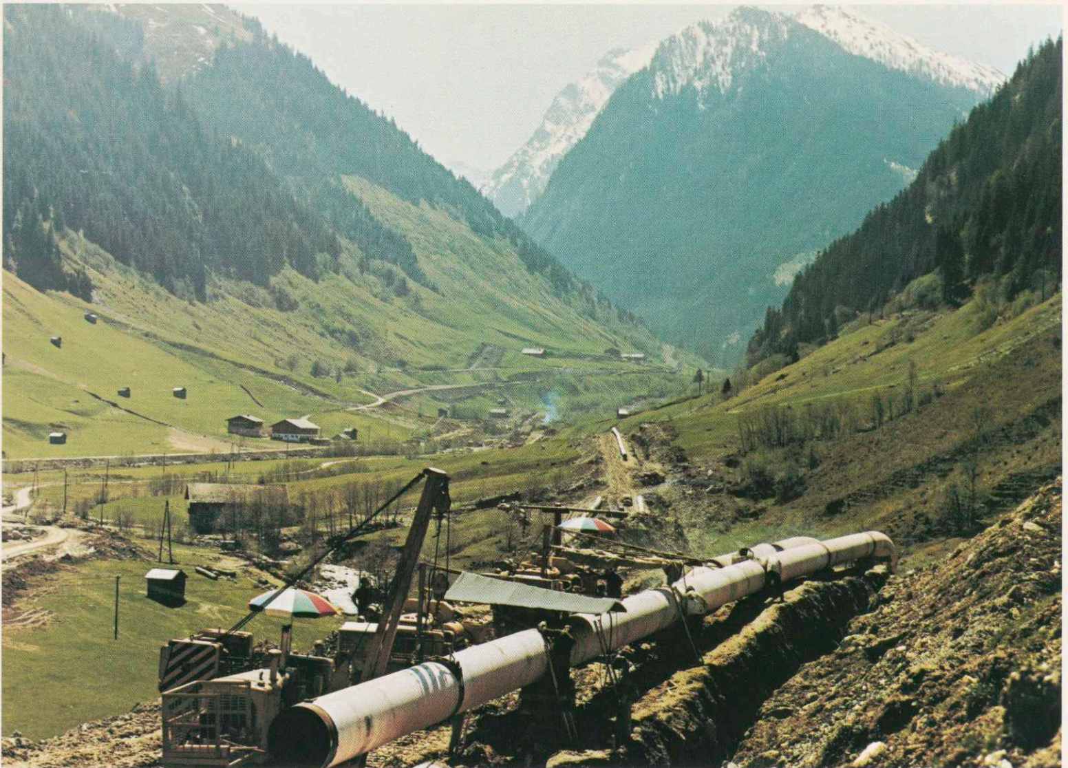
A 287-mile petroleum pipeline system from northern Italy through the Austrian Alps to West Germany includes marine terminal, tank farm and pumping stations.
