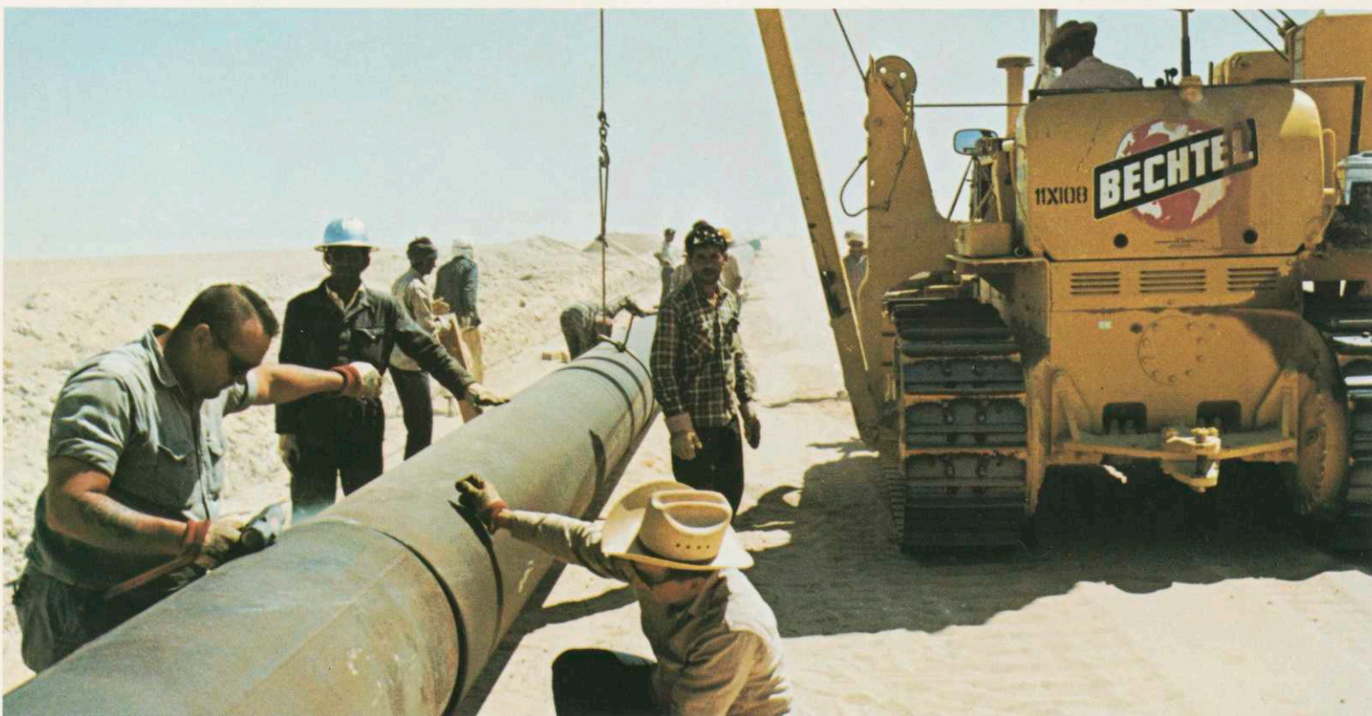
Company equipment is used on remote projects worldwide, such as this north African pipeline project.
