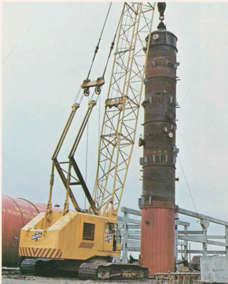
Bechtel's equipment performing a lift at a refinery project in Wales, helped complete the 100,000-barrels-per-day project in 20 months from groundbreaking.
