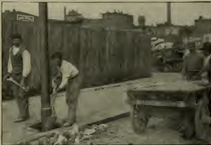
PUTTING IN CONCRETE AT THE BASE OF THE RECLAIMED POLE. THE PORTABLE CONCRETE MIXER IS SHOWN AT THE RIGHT
