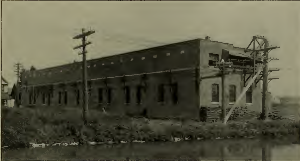
TERMINAL HOUSE OF THE CATARACT POWER & CONDUIT COMPANY. THREE 22,000-VOLT LINES ENTER AT THE WEST END, AND THE 2200-VOLT LINES LEAVE THE BUILDING ALONG THE NORTH WALL, PASSING UNDER THE 22,000-VOLT LINES AND EXTENDING SOUTHWARD ALONG THE ERIE CANAL, SEEN IN THE FOREGROUND, TO MANUFACTURING PLANTS IN NORTH BUFFALO
