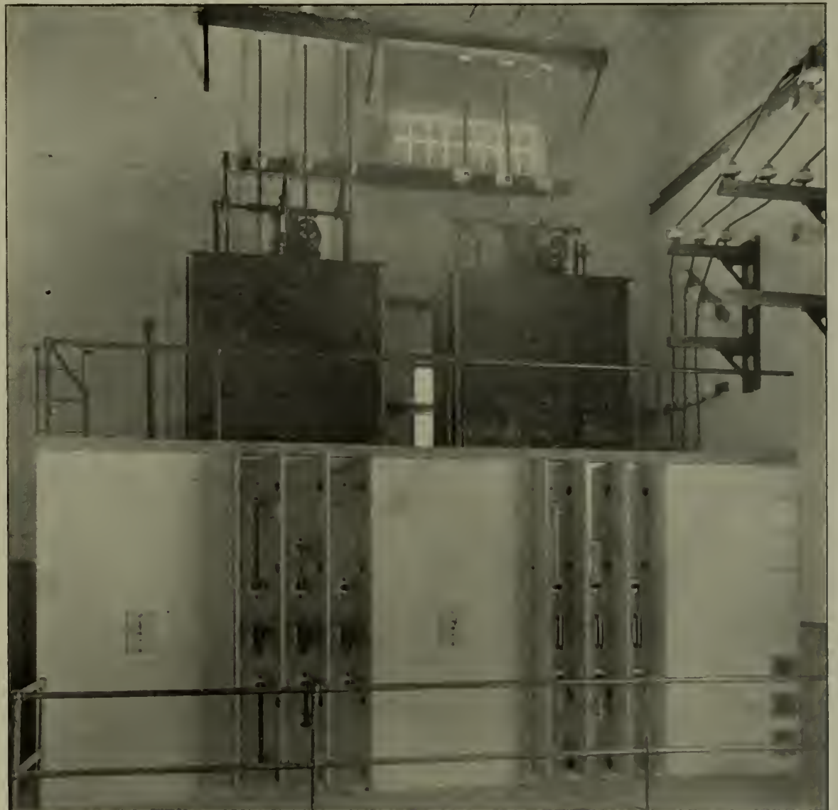
THE EAST END OF THE TERMINAL HOUSE, SHOWING SELECTOR SWITCHES AND 22,000-VOLT OIL SWITCHES FOR TRANSFORMERS
