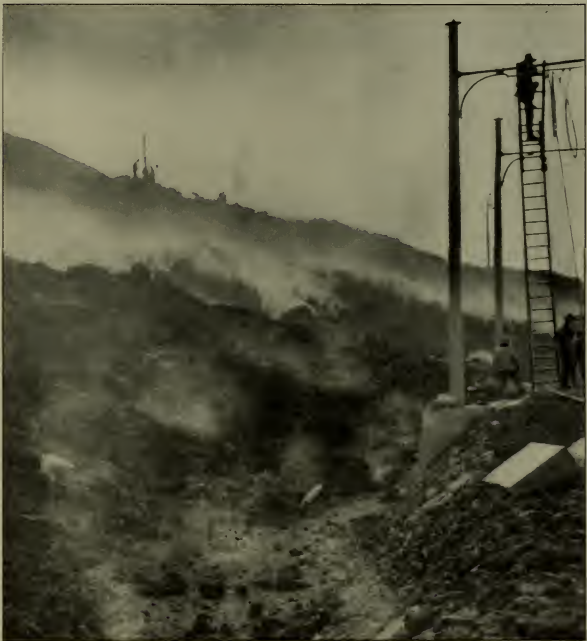
RECONSTRUCTING A PART OF THE VESUVIUS ELECTRIC RAILWAY DESTROYED DURING THE ERUPTION OF JANUARY. THE VAPOUR IS FROM THE HOT LAVA
