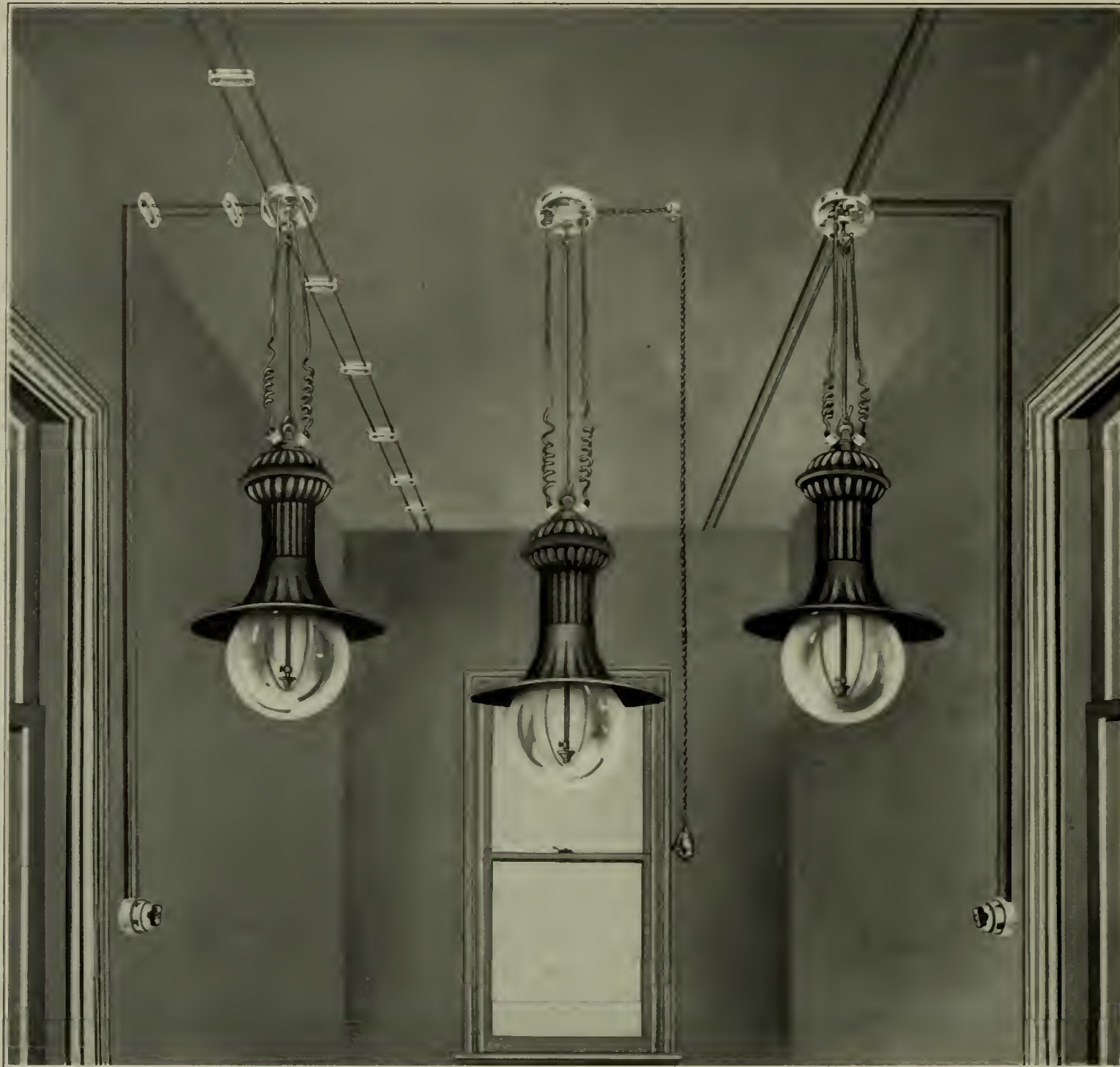
FIG. 4.—THE THREE DIFFERENT STYLES OF PAISTE HANGER BOARDS FOR MULTIPLE ARC LAMPS APPLIED TO THEIR RESPECTIVE METHODS OF WIRING
