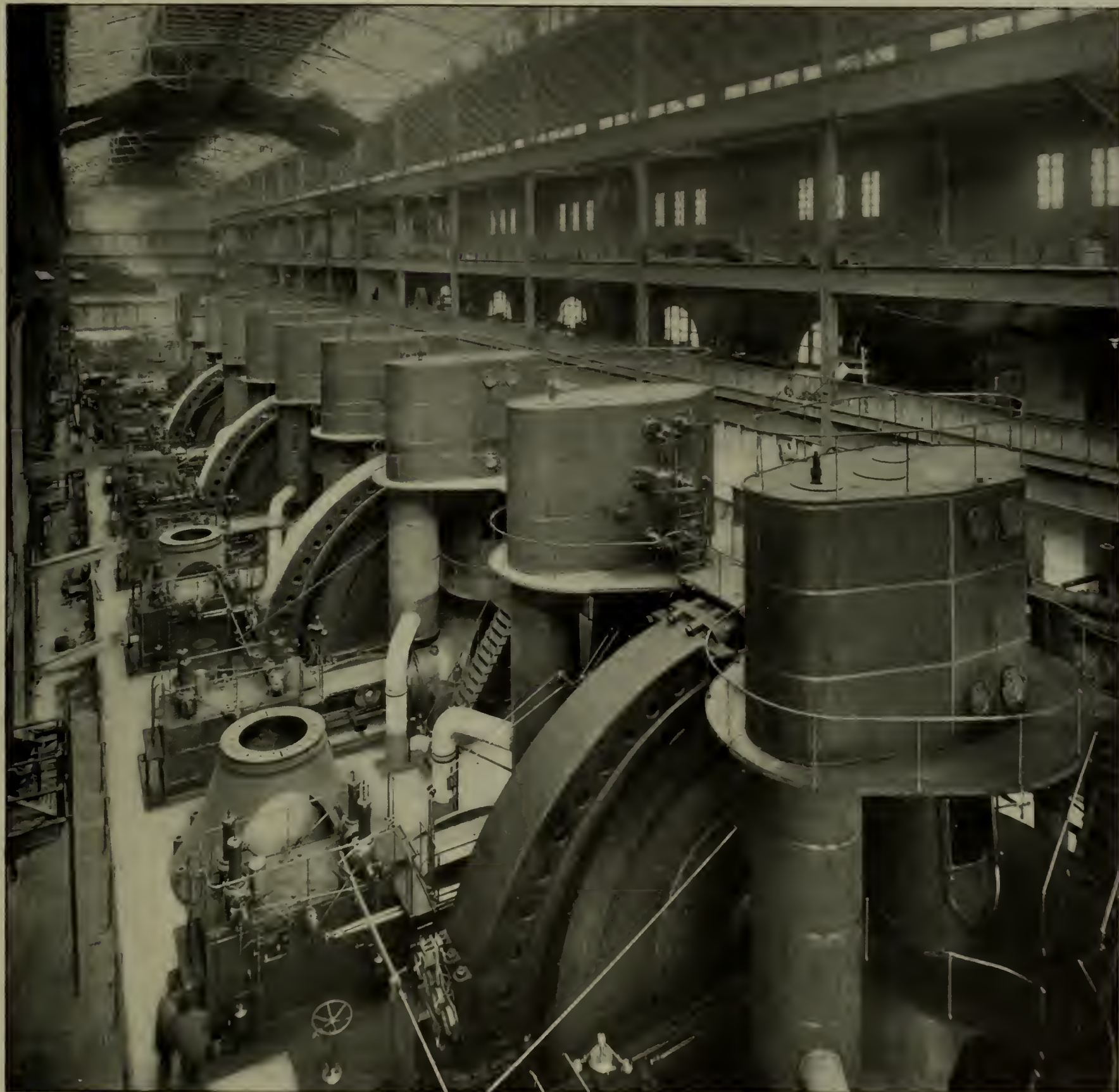
THE FIFTY-NINTH STREET STATION OF THE INTERBOROUGH RAPID TRANSIT COMPANY, NEW YORK, SHOWING REYNOLDS-CORLISS ENGINES BUILT BY THE ALLIS-CHALMERS COMPANY, MILWAUKEE, WIS.
