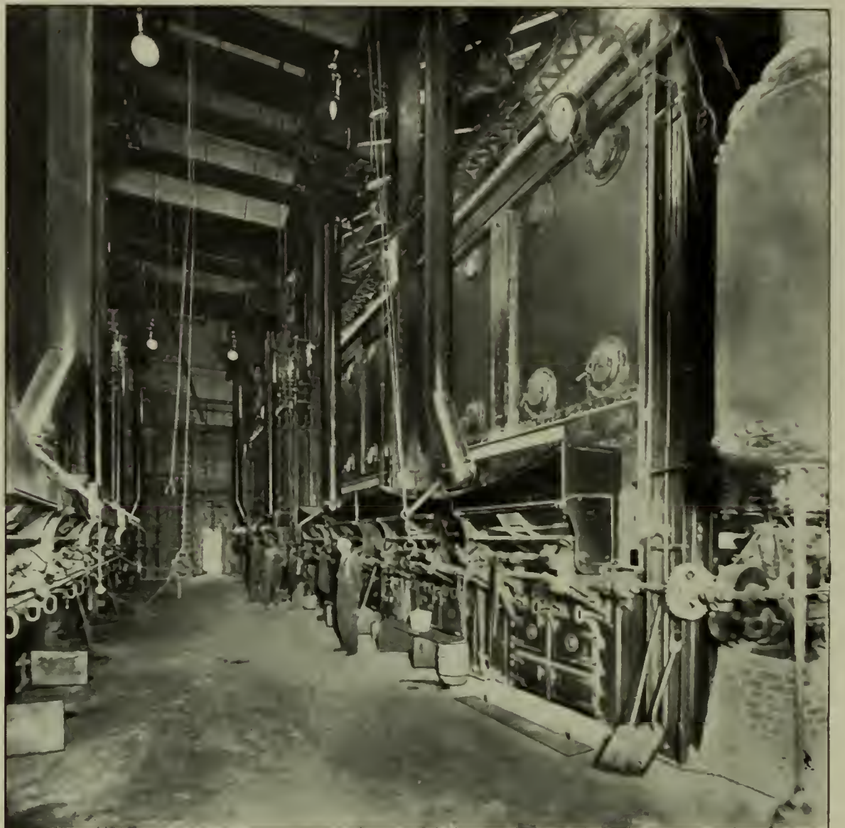
THE BOILER ROOM IN THE GOULD STREET STATION OF THE MARYLAND TELEPHONE COMPANY
