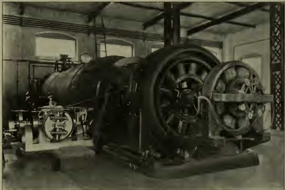
INTERIOR OF THE POWER HOUSE, SHOWING A 300-KW. UNIT AND EXCITER. THE GOVERNOR SHOWN IN THE ILLUSTRATION ABOVE IS ALSO SHOWN HERE
