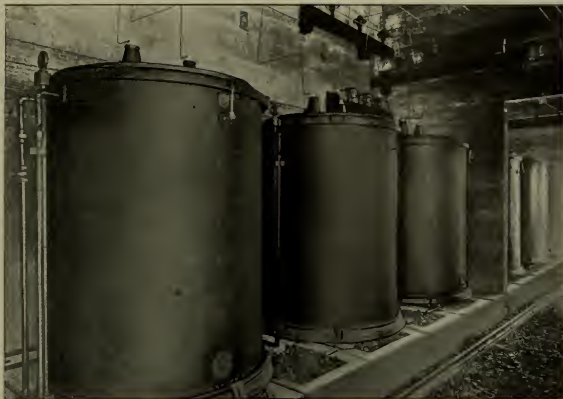
THE 300-KW. BULLOCK TRANSFORMERS ARE OF THE OIL-FILLED, WATER-COOLED TYPE, STEPPING UP FROM 2200 TO 19,050 VOLTS. THEY ARE CONNECTED IN DELTA ON THE LOW-VOLTAGE SIDE, AND IN Y ON THE HIGH-VOLTAGE SIDE, GIVING A LINE POTENTIAL OF 30,000 VOLTS
