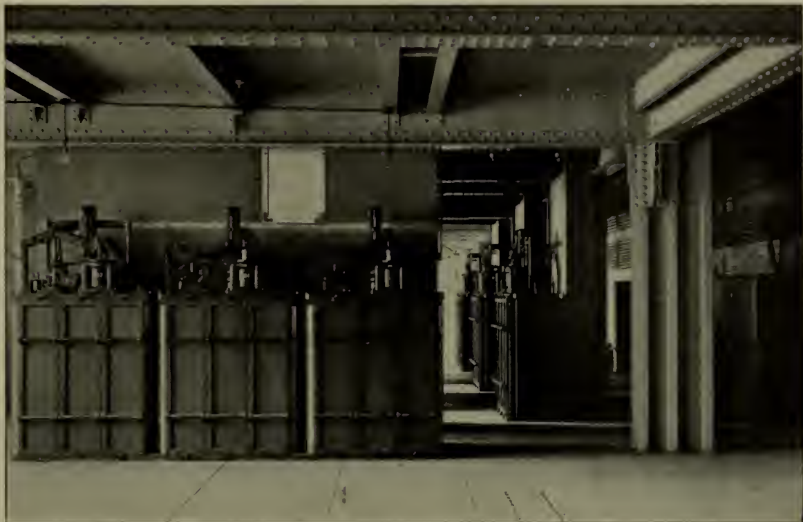
THE FEEDER GALLERY, SHOWING THE OIL CIRCUIT BREAKERS FOR FEEDERS AND GENERATORS
