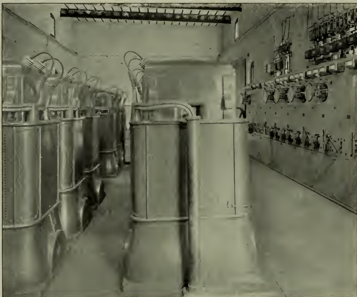
TRANSFORMERS AND 11,000-2200-VOLT SWITCHBOARD IN STATION NO. 4. THE SERIES AND POTENTIAL TRANSFORMERS FOR THE INSTRUMENTS ARE MOUNTED ON THE WALL
