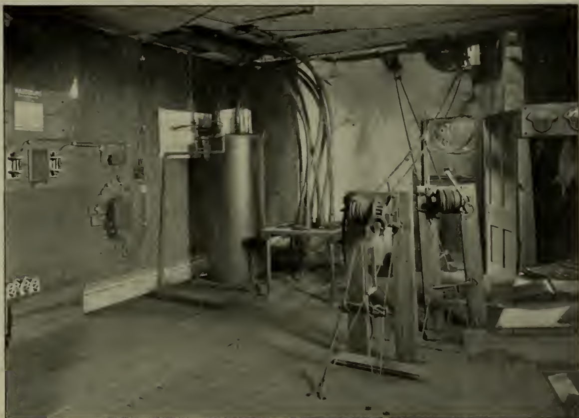
THE TRANSFORMER ROOM. THE CURRENT IS STEPPED DOWN FROM 2200 VOLTS TO 20, 80 OR 100 VOLTS OR MORE
