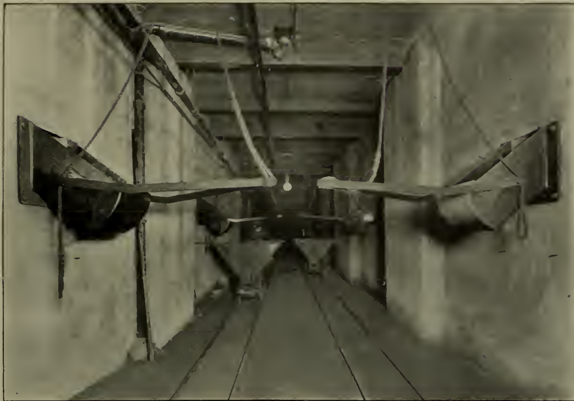
THE ASH-HANDLING MACHINERY IN THE GOULD STREET STATION OF THE MARYLAND TELEPHONE COMPANY
