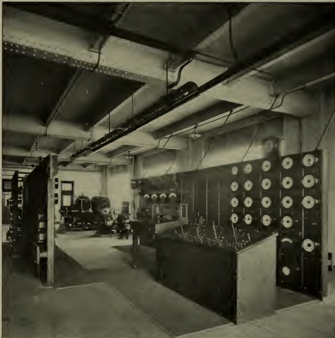
THE ELECTRICAL OPERATING GALLERY, SHOWING THE MOTOR-DRIVEN EXCITER, INSTRUMENT BOARD, AND SWITCHBOARD
