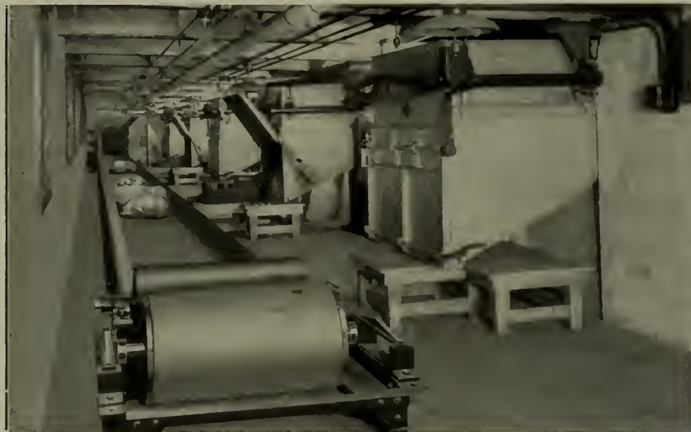
THE MAIL-HANDLING MACHINERY IN THE NEW CHICAGO POSTOFFICE IS MOTOR-DRIVEN, AND WAS INSTALLED BY THE JEFFREY MANUFACTURING COMPANY, OF COLUMBUS, OHIO. THE WEIGHING HOPPERS AND CONVEYORS IN THE BASEMENT ARE SHOWN HERE
