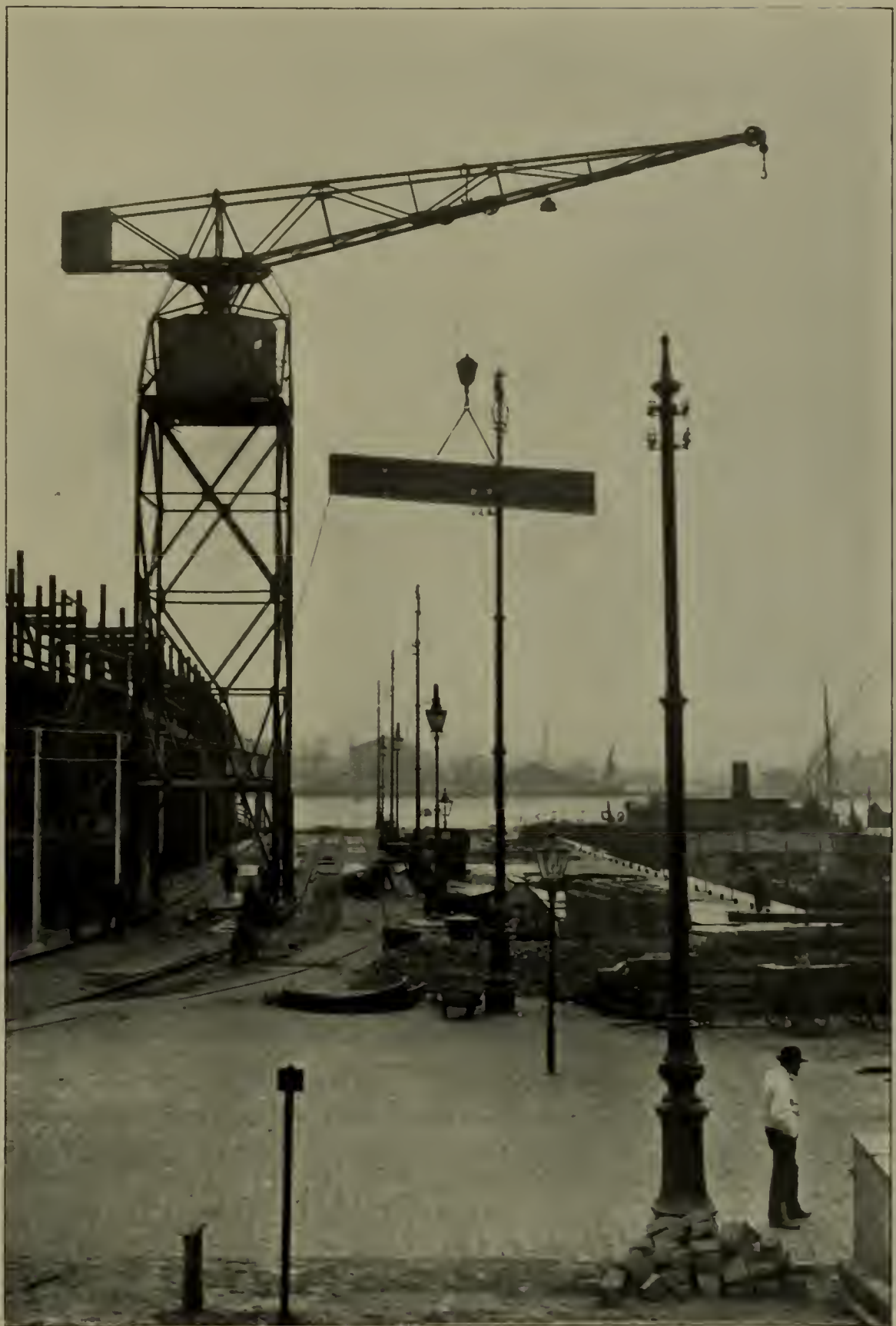
FIG. 15.—A ROTARY TOWER CRANE AT THE IMPERIAL SHIP WORKS, WILHELMSHAVEN. CURRENT IS SUPPLIED TO THE CRANE BY THE FEED WIRES SHOWN AT THE LEFT, EXTENDING ALONG THE RUNWAY AND SUPPORTED ON POLES
