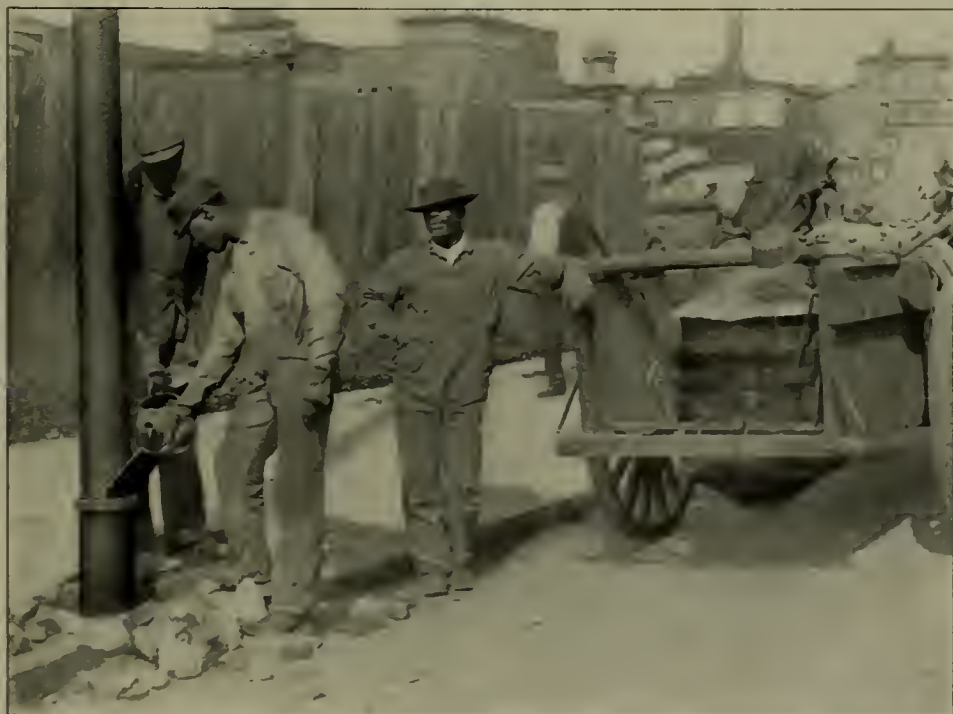
POURING IN SULPHUR AROUND A REINFORCING SLEEVE MADE BY WILLIAM D. GHERKY, PHILADELPHIA. THE WAGON FOR MELTING THE SULPHUR IS SHOWN AT THE RIGHT
