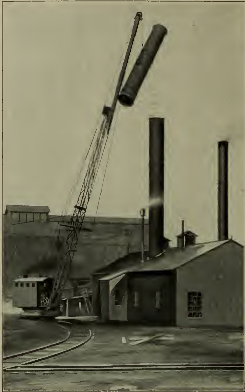
A LOCOMOTIVE CRANE BUILT BY THE BROWNING ENGINEERING COMPANY, CLEVELAND, OHIO, CARRYING A SECTION OF A SMOKE-STACK WEIGHING 4\frac{1}{2} TONS, AT A RADIUS OF 25 FEET
