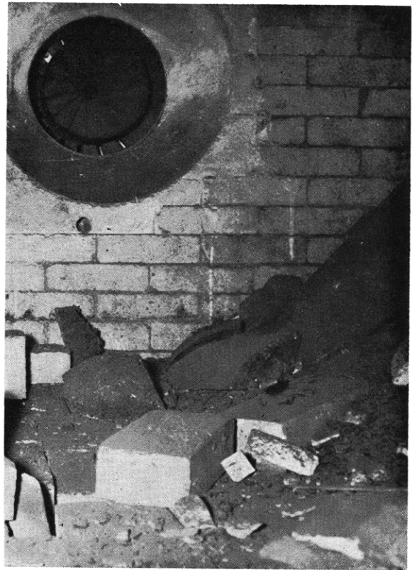
Fig. 38 Dislodged boiler brickwork
