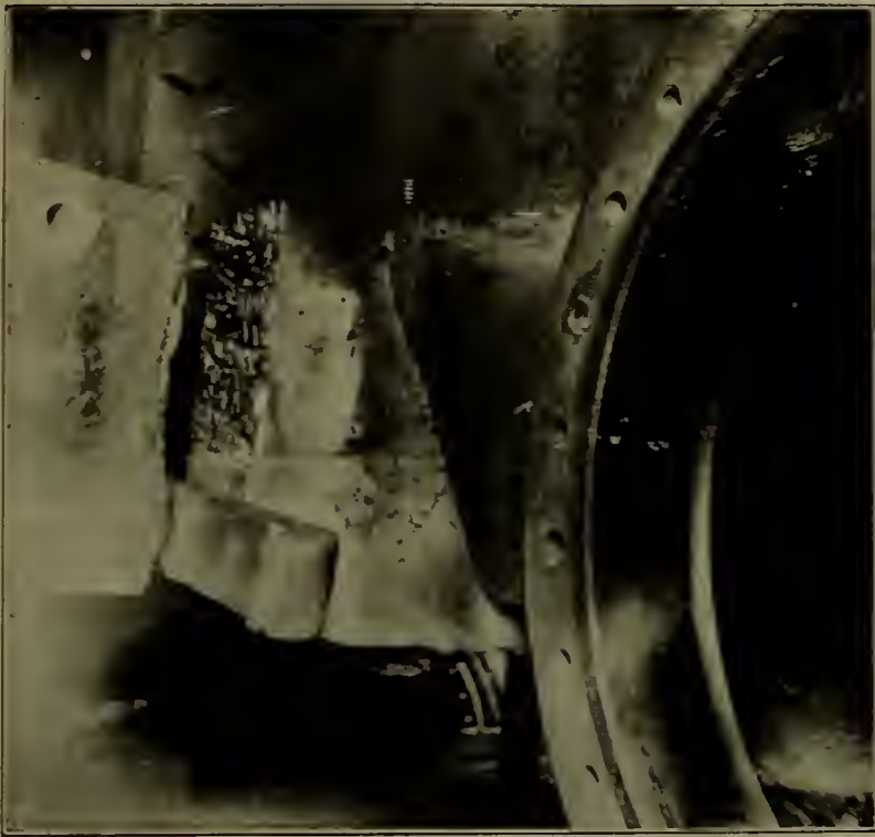
Frame of Engine 1057, Broken Behind Cylinders, Cut and Ready for Welding.
