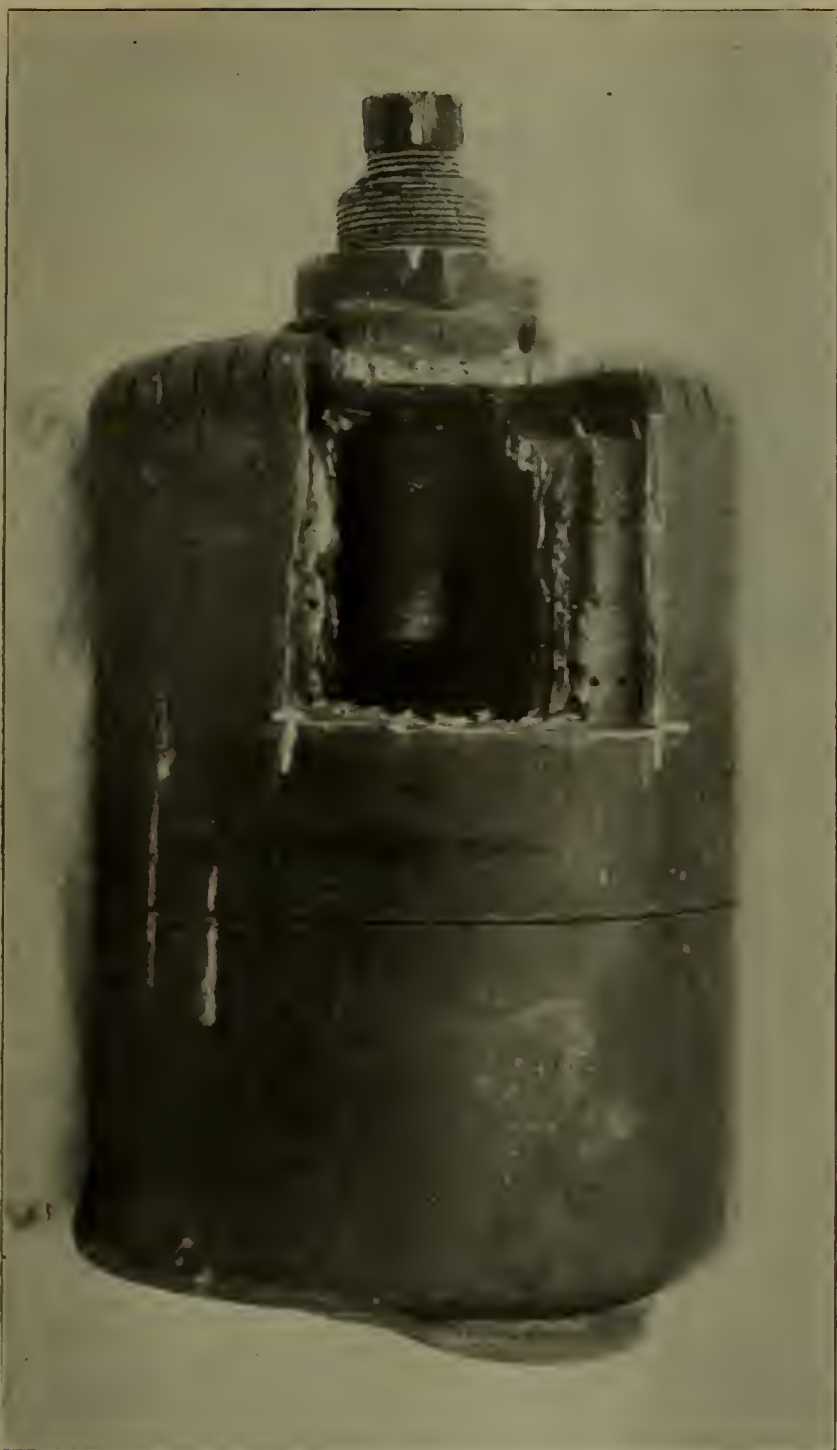
Safety Valve Casing Showing Condition of Adjusting Screws. This Valve Caused an Explosion.
