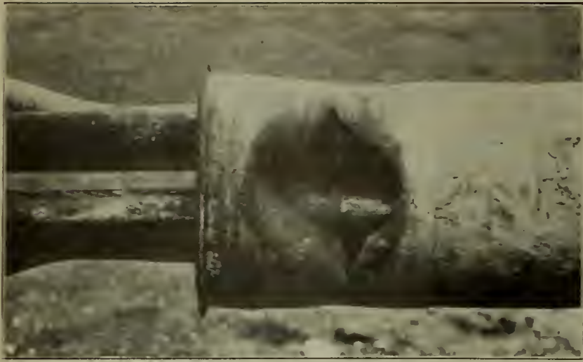
Showing the Collapse of a Superheater Tube.
