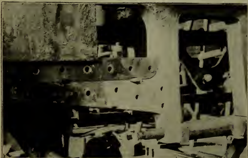
Broken Splice Leg Welded by Oxy-Acetylene.
