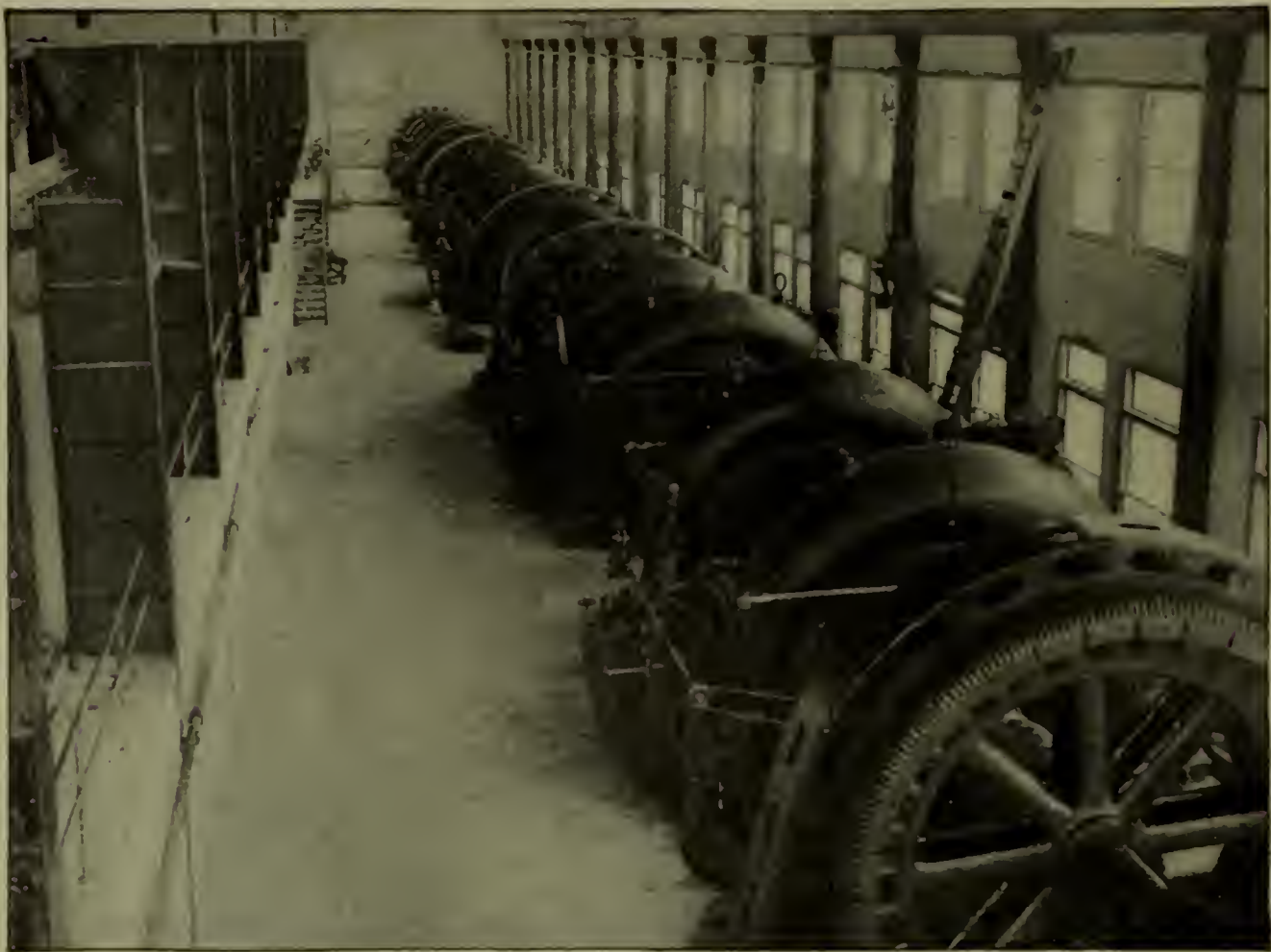
Interior of Generator Room in the Rainbow Station of the Great Falls Power Co., Containing Six 6,000-H. P. Units.
