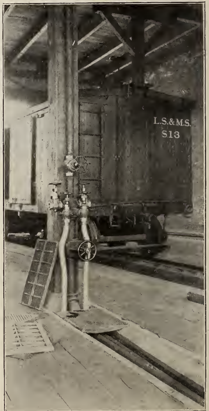
FIG. 7—"MIXING BOX," ELKHART ROUNDHOUSE.
