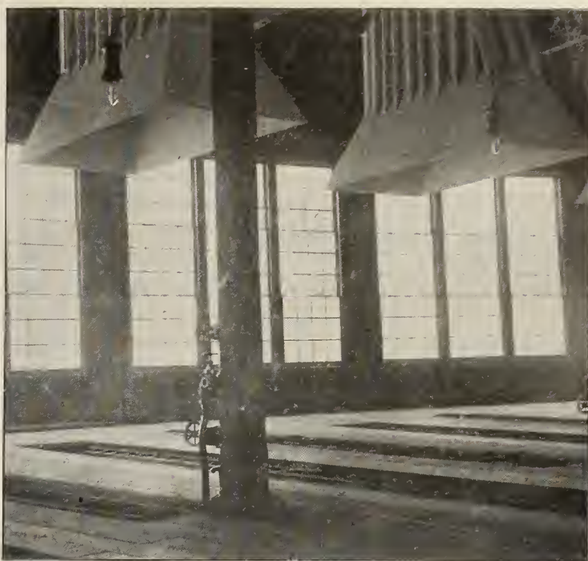
FIG. 8—INTERIOR VIEW, SHOWING WINDOWS IN OUTER WALL AND BOTTOM OF JACK, ELKHART ROUNDHOUSE.
