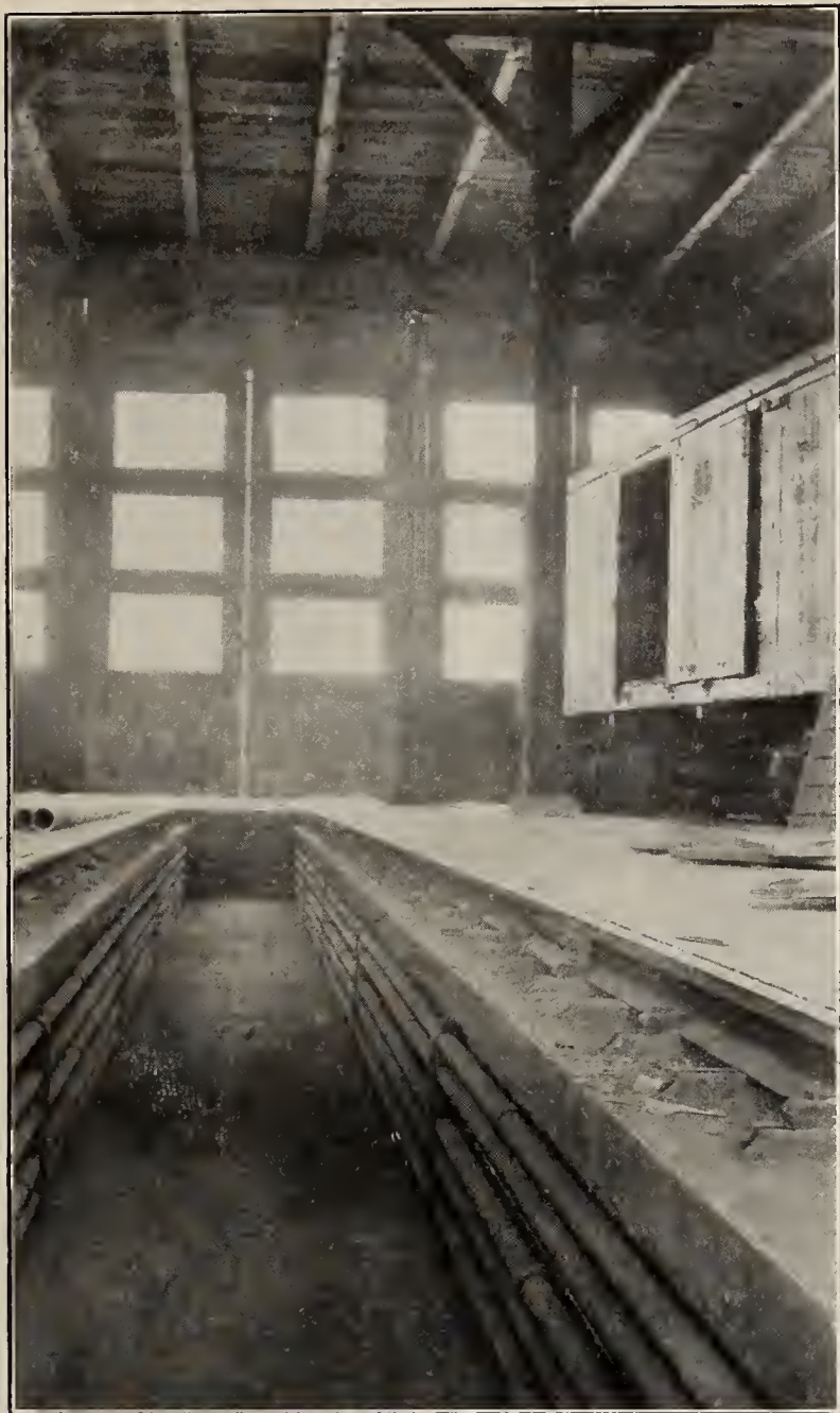
FIG. 8—HEATING PIPES IN PIT, CAST IRON COPING FOR PIPES AND WINDOWS IN DOORS, ELKHART
