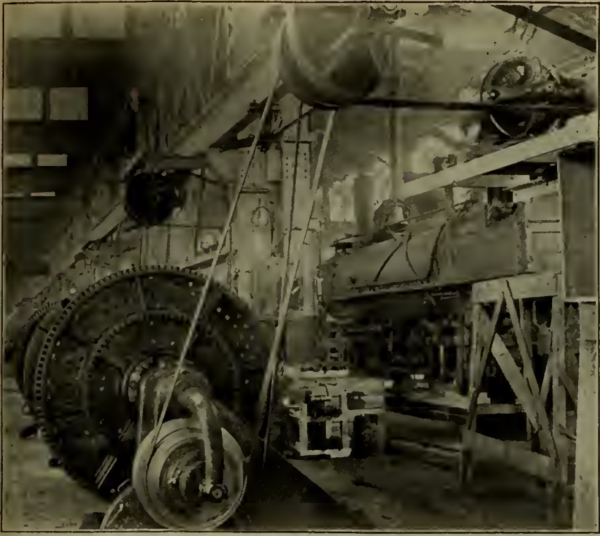
FIG. 9—TOPEKA SHOPS OF THE ATCHISON, TOPEKA & SANTA FE RAILWAY—SHOWING BELT CONNECTION TO 74-IN. SELLERS LATHE OPERATED BY A 7\frac{1}{2} H. P. GENERAL ELECTRIC MOTOR.
