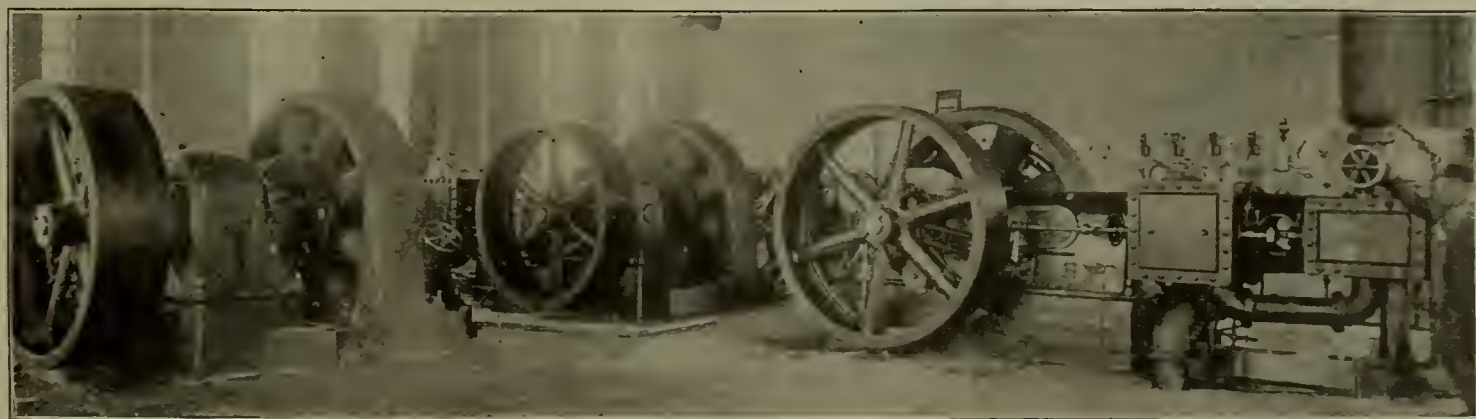
FIG. 4—TOPEKA SHOPS OF THE ATCHISON, TOPEKA & SANTA FE RAILWAY—GENERATING UNITS.
