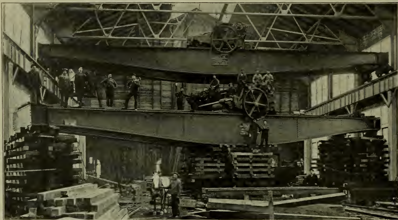
ELEVATION OF TRAVELING CRANES WITH JACKS, AT THE FORT WAYNE SHOPS OF THE PENNSYLVANIA LINES.
