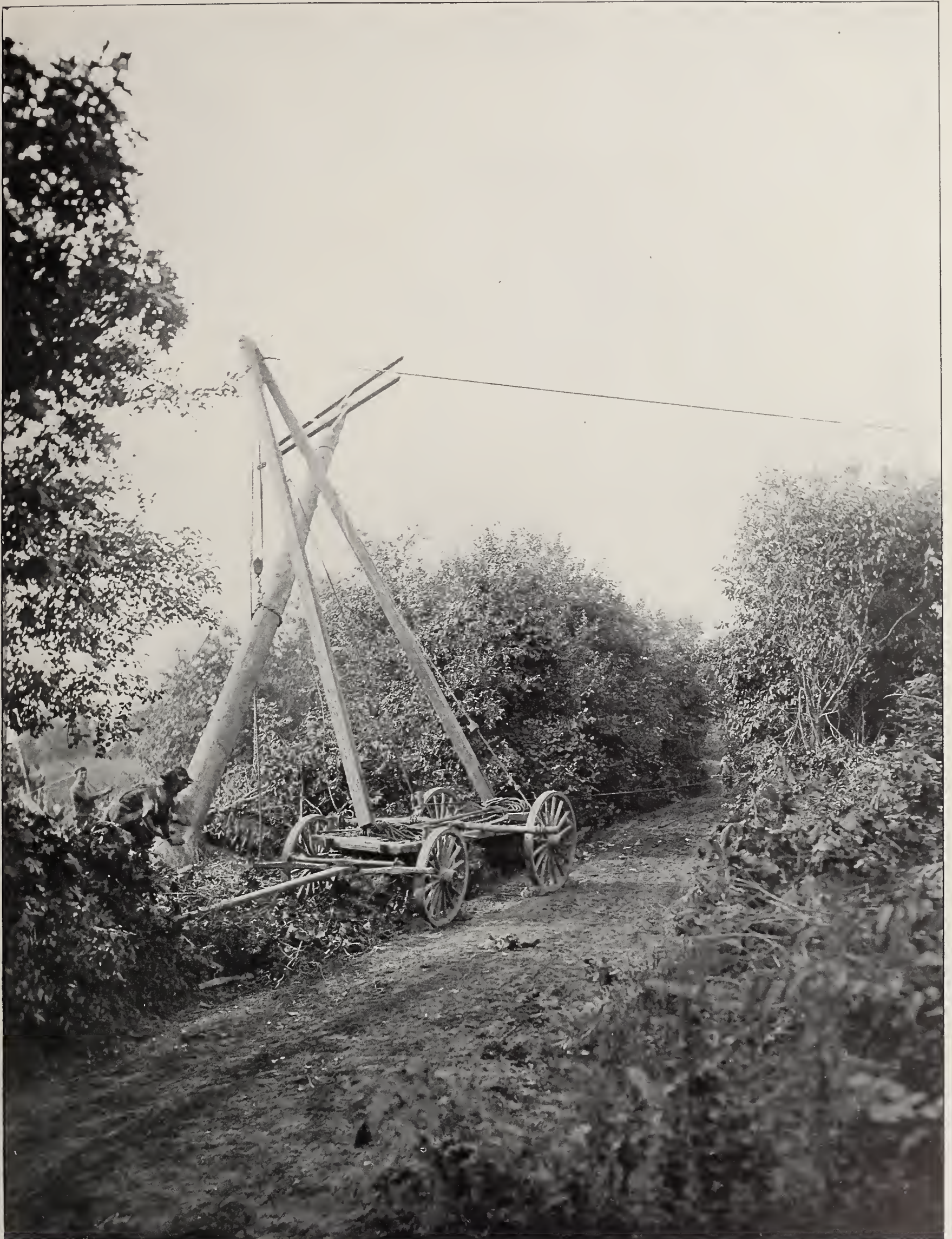
FIG. 4.—RAISING POLES BY DERRICK. FORMERLY TWENTY MEN WERE REQUIRED TO RAISE A POLE. NOW FIVE MEN AND TWO HORSES DO THE WORK
