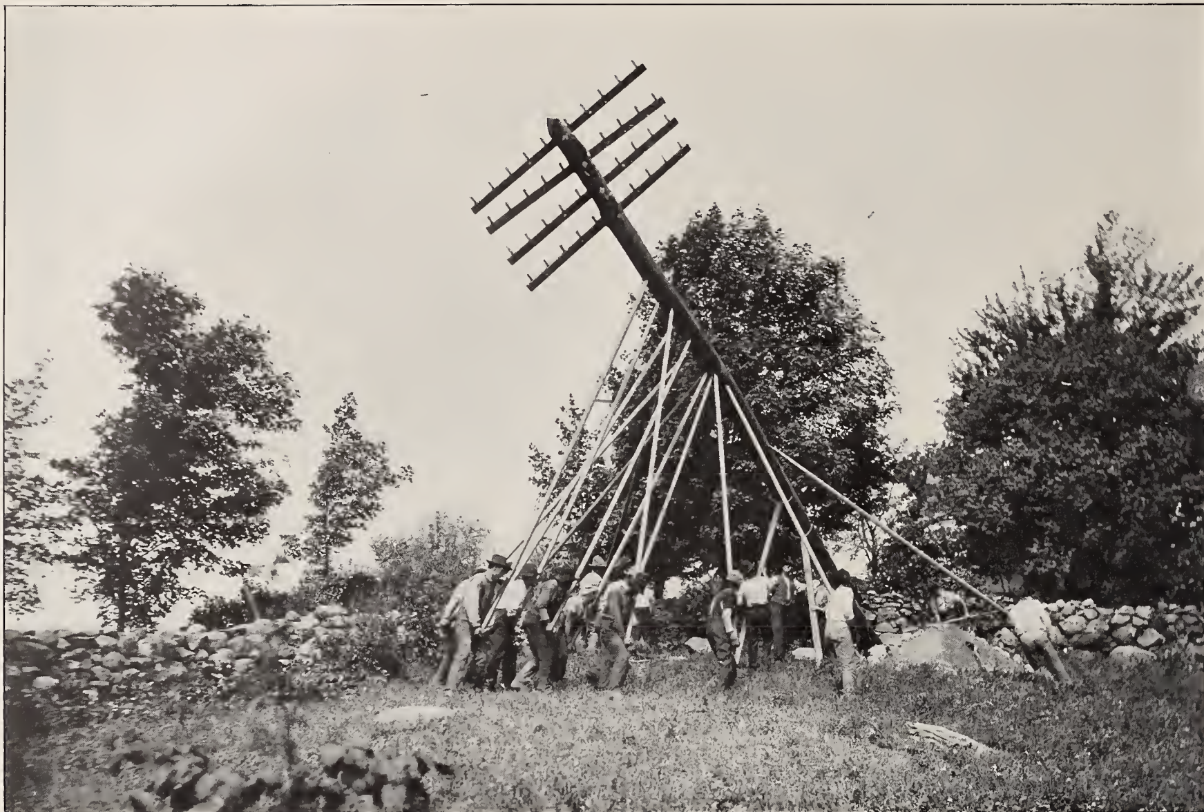
FIG. 2.—THE OLD WAY OF RAISING A POLE. THE SAVING IN MEN REQUIRED BY USING A DERRICK MAY BE CLEARLY SEEN BY COMPARING THIS WITH THE METHOD ILLUSTRATED IN FIG. 4
