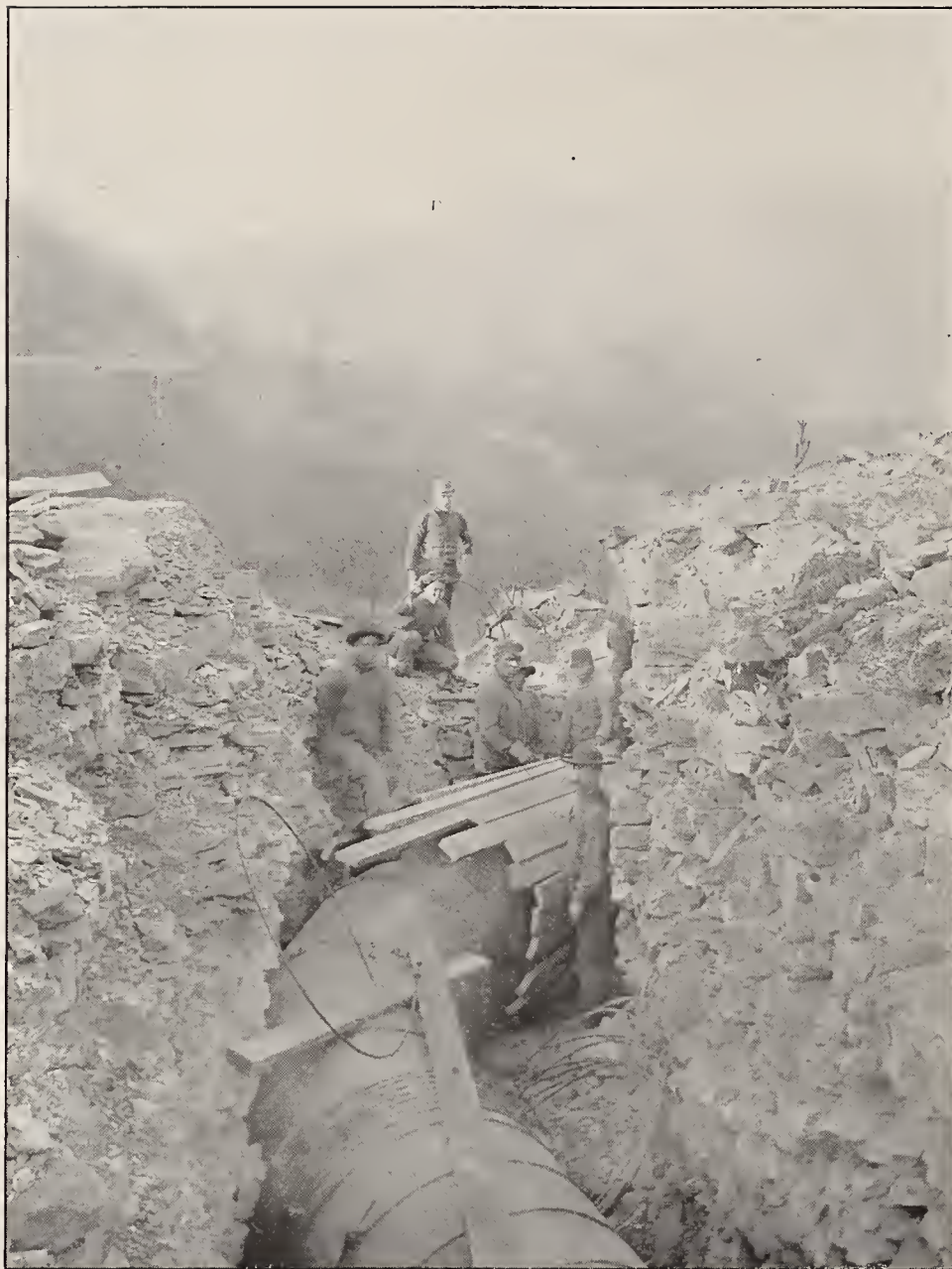
FOR SHARP CURVES A STEEL ELBOW IS SOMETIMES USED, BUT IN ORDINARY CASES THE WOODEN STAVE PIPE IS SPRUNG TO THE DESIRED DEGREE
