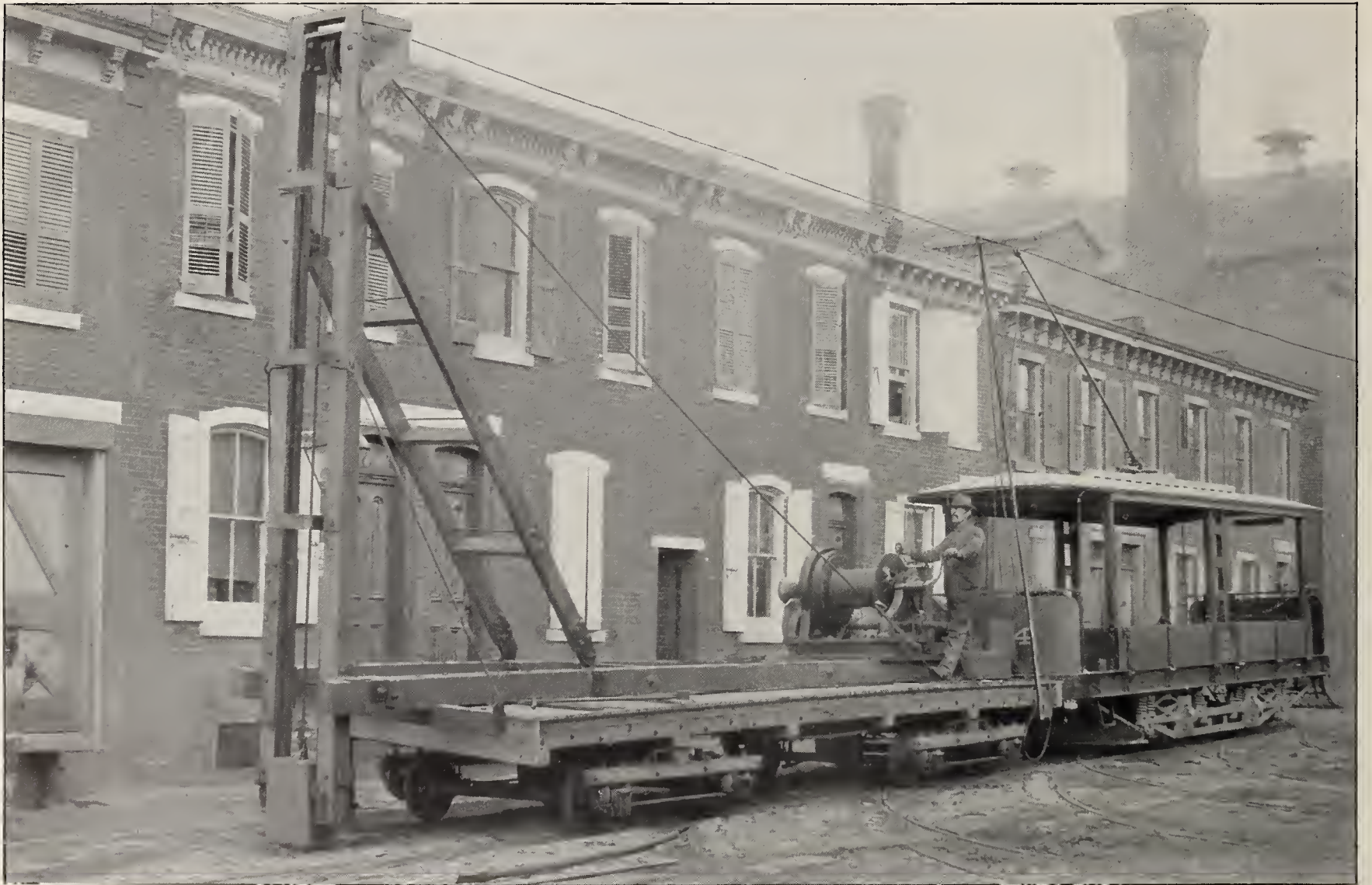
A PORTABLE ELECTRICALLY DRIVEN DROP HAMMER, SHOWN BOTH ERECTED, READY FOR WORK, AND DISMANTLED FOR TRANSPORT. OPERATING CURRENT IS HERE ALSO TAKEN FROM THE TROLLEY WIRE BY FISH-POLE CONNECTION, AS SHOWN
