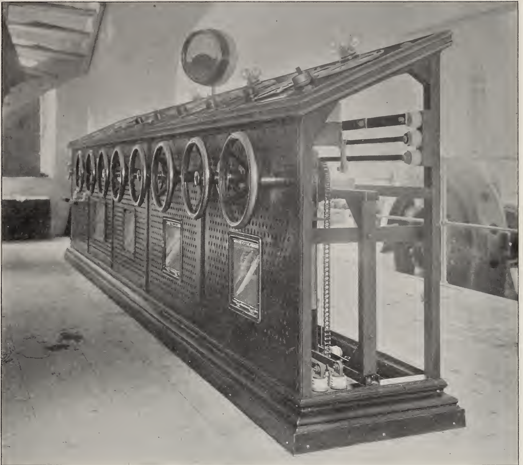
THE MAIN OPERATING BOARD
