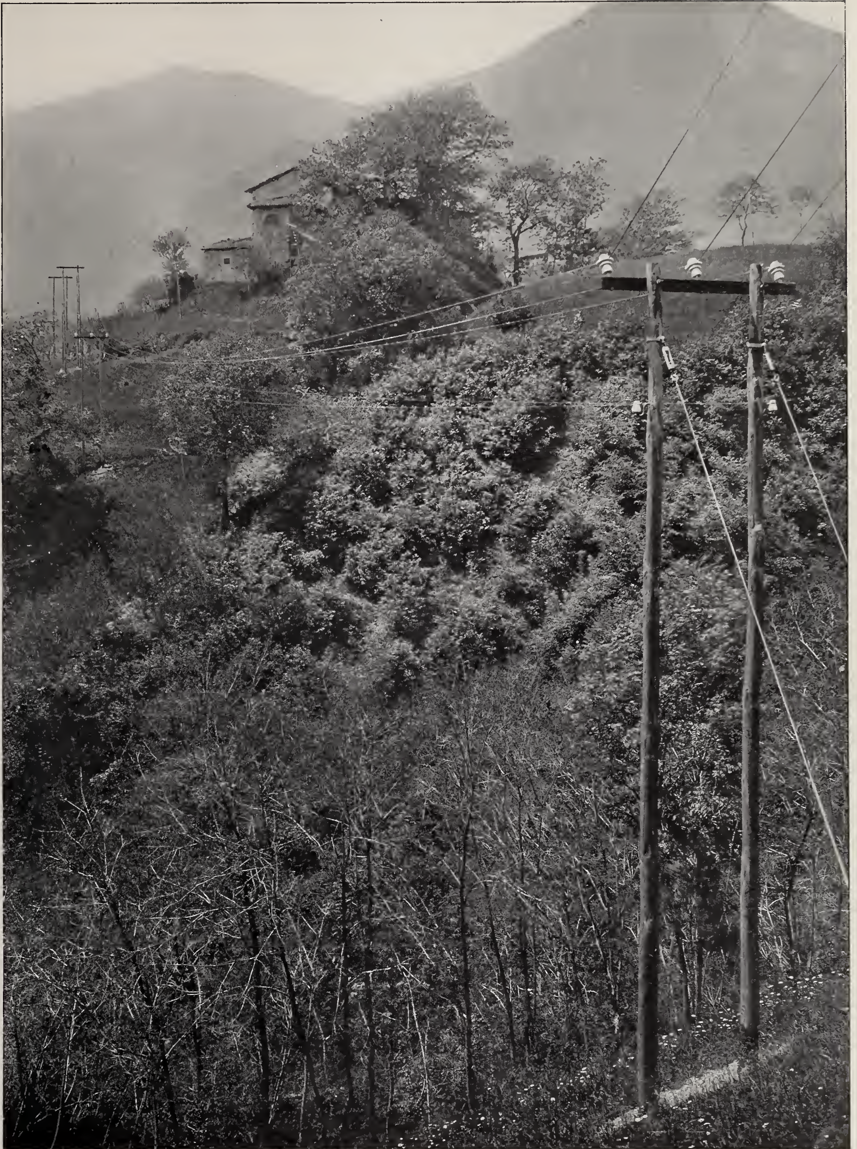
A PORTION OF THE TRANSMISSION LINE
