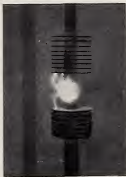
FIG. 9.—DISCHARGE OF THE 20-K. W. TRANSFORMER IN THE DE FOREST ST. LOUIS EXPOSITION STATION. SPARK GAP ONE INCH. SEE PAGE 163
