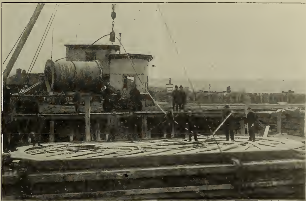
Transferring the Cable from the Reels to the Deck of the Wrecking Scow.
